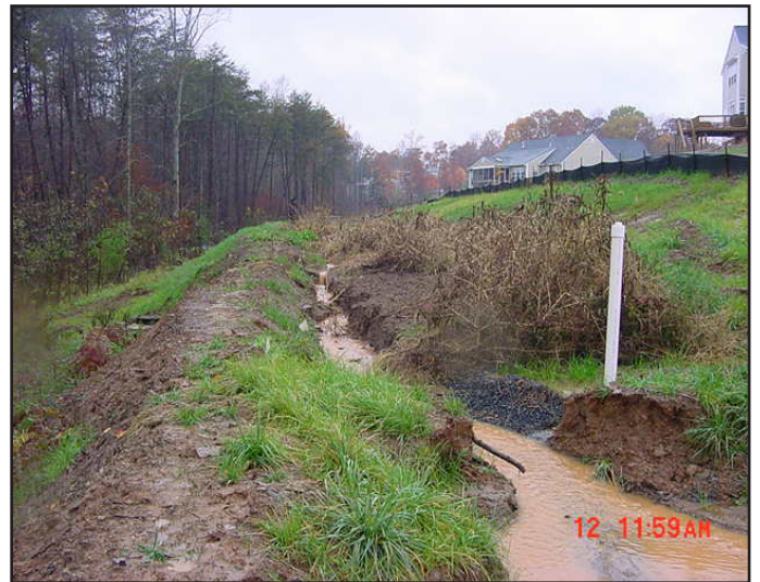
A major issue with conversions is timing. Premature installation of the post-construction practice can result in damage from construction sediments.
