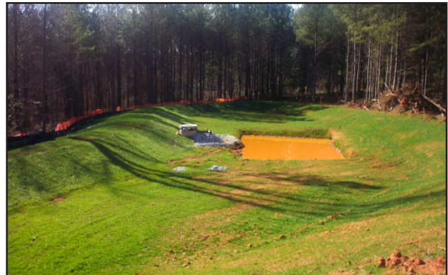
Figure 2.10 - Storm water detention structures will reduce storm water runoff from developed areas.
