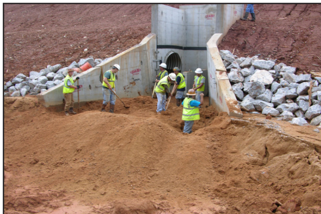
Figure 1.2 - Maintaining outlet protection due to BMP failures higher in the drainage basin.
