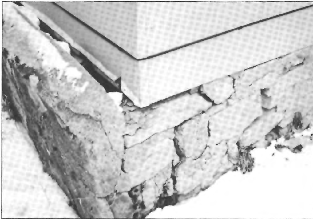
Figure 304.5 MAJOR DAMAGE TO A FOUNDATION WALL This foundation is crumbling. Failure to repair it will eventually lead to its collapse.
